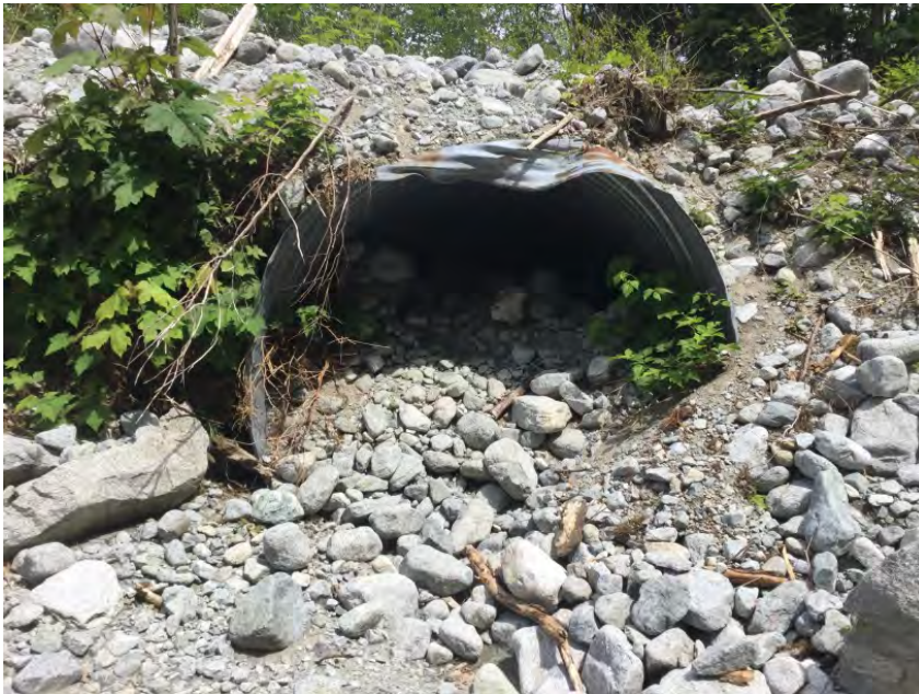
High chain inlet 67% plugged from recent event
