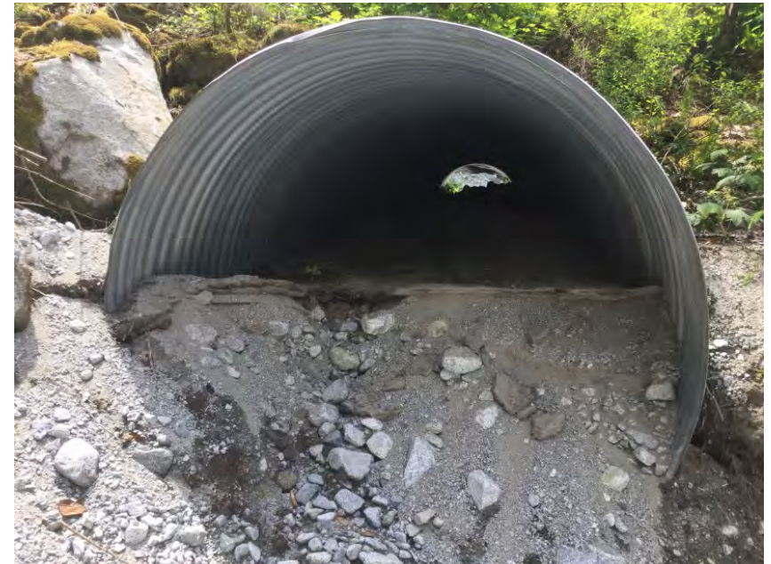
High chain culvert 50% plugged
