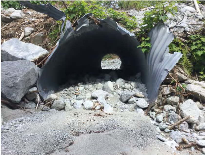
Low chain inlet damage from recent event
